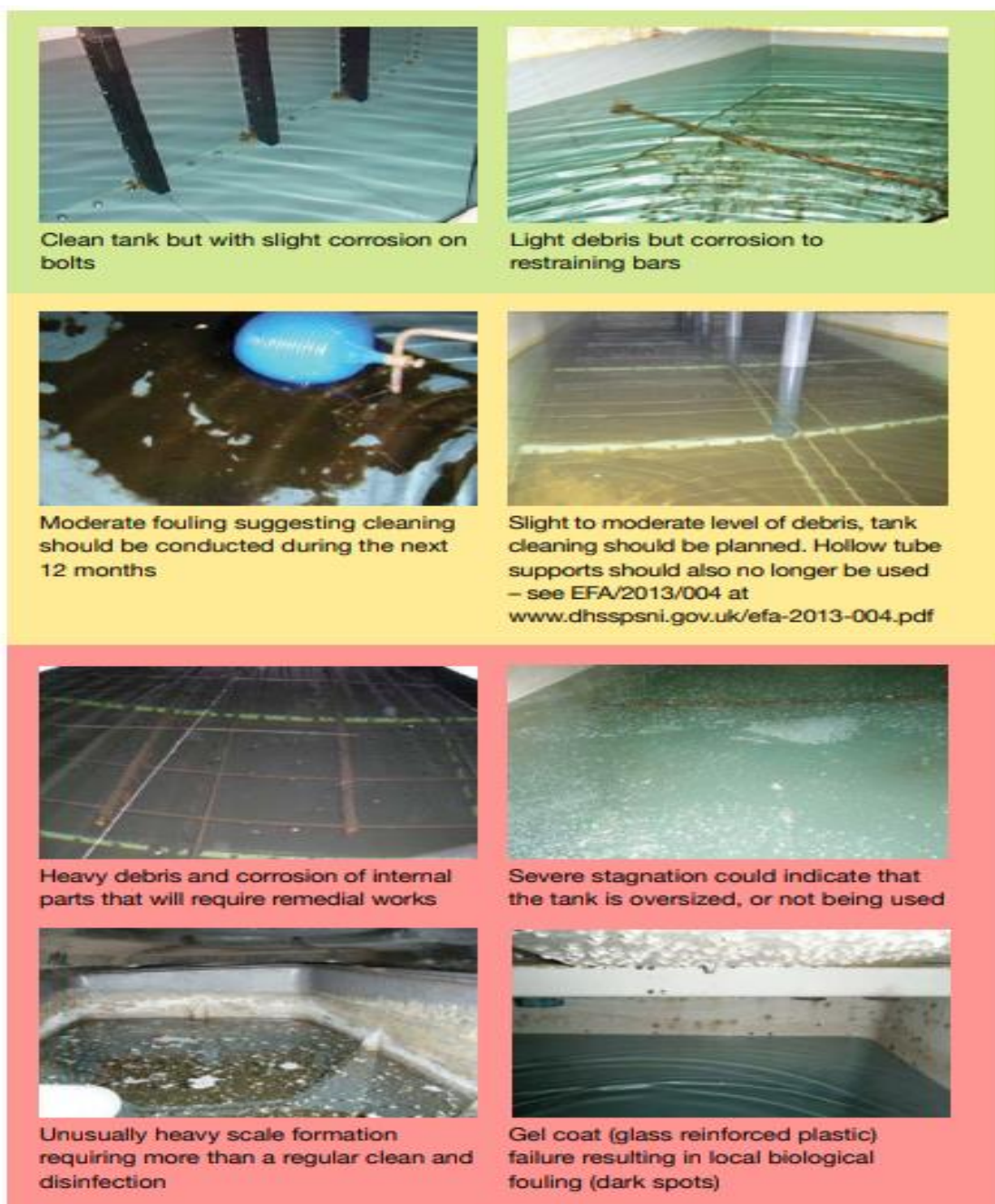
Figure 13 Illustration of cold water storage tanks in various conditions set against traffic light colour coding.
