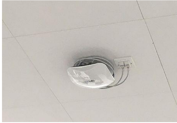
Figure 15.9:1 AP installation on suspended modular ceiling
