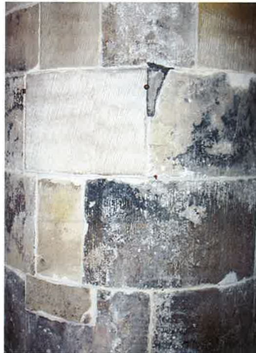
Pillar built of sandstone blocks showing examples of both original stones (dark grey) and 1909 renovations (paler).
